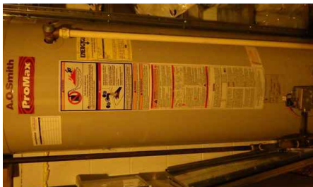
50 gallon gas hot water heater.
