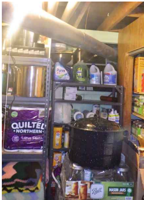
Storage units blocking view of foundation wall.
