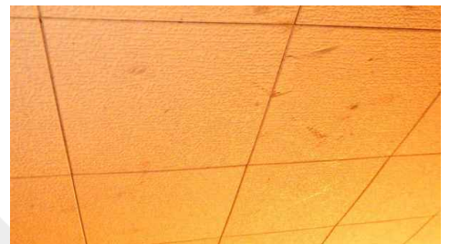
Dents in ceiling tile near stairwell.
