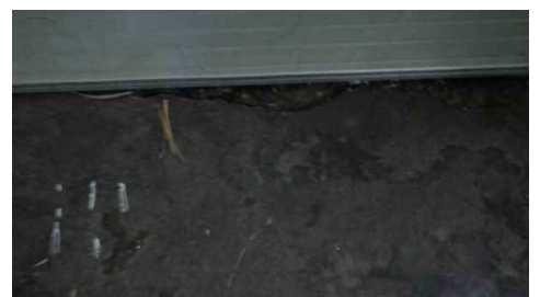
Some cracking of tile near egress door.
