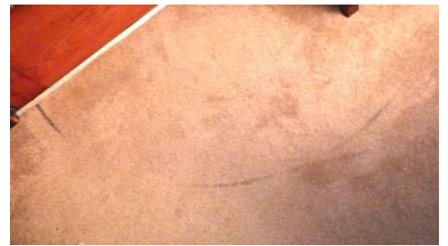
Front door carpet, line from door dragging on floor.
