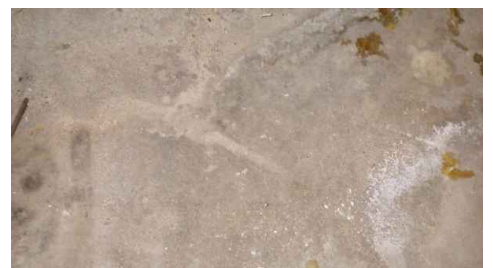
Efflorescence observed under ductwork.
