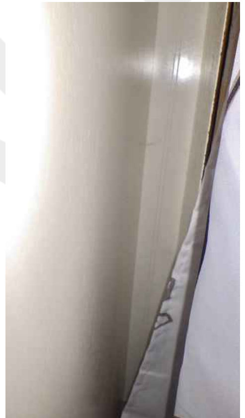
Access panel for shower has been sealed off and mostly covered by cabinet.
