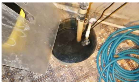
Sump well with submersed pump.
