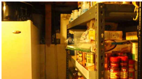
Storage units blocking view of foundation wall.
