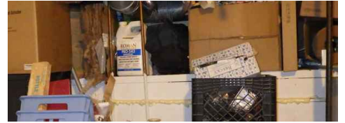
Personal items blocking entry into crawlspace from sump room.
